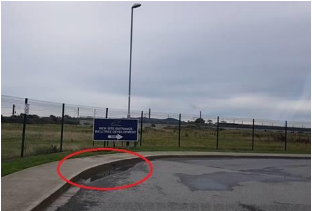
Figure 7: Ponding in carriageway
